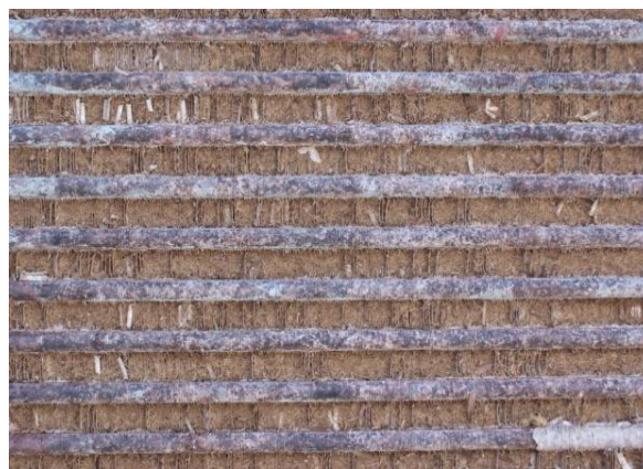
Figure 2: Damaged and blocked condenser
