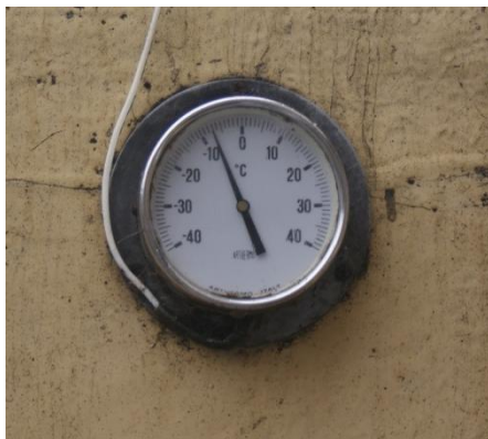
Figure 14: Brine tank temperature setting
