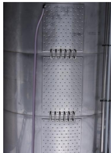
Figure 12: Uninsulated wine tank with brine jacket for cooling
