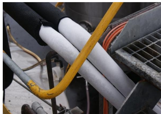
Figure 13: Missing insulation on brine lines
