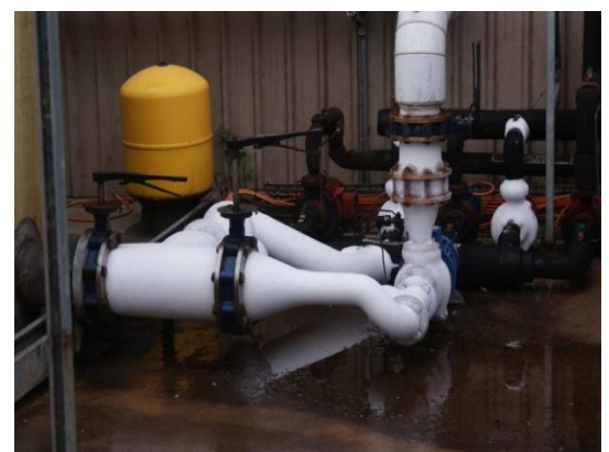
Figure 11: Icing up of brine pumps and lines
